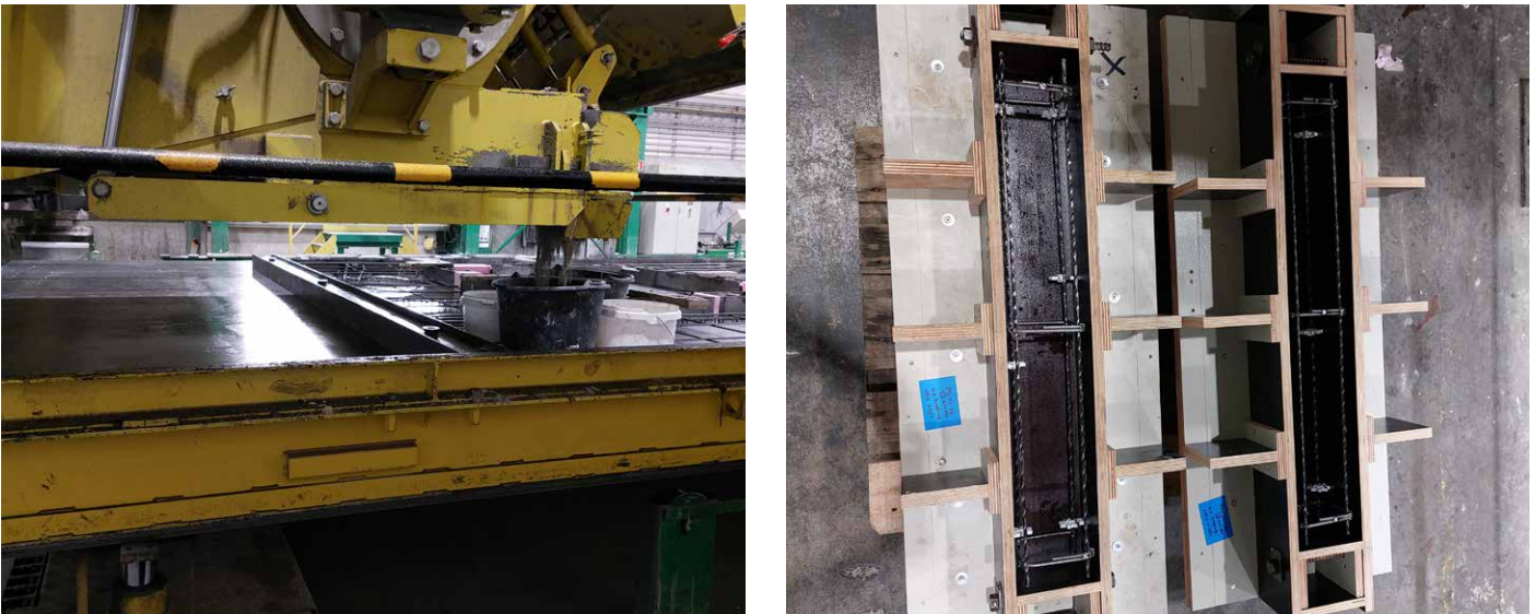
Figure 2: Pouring concrete from the pouring machine at the company of Voorbij Prefab (left) and moulds with basalt rebar (right)
